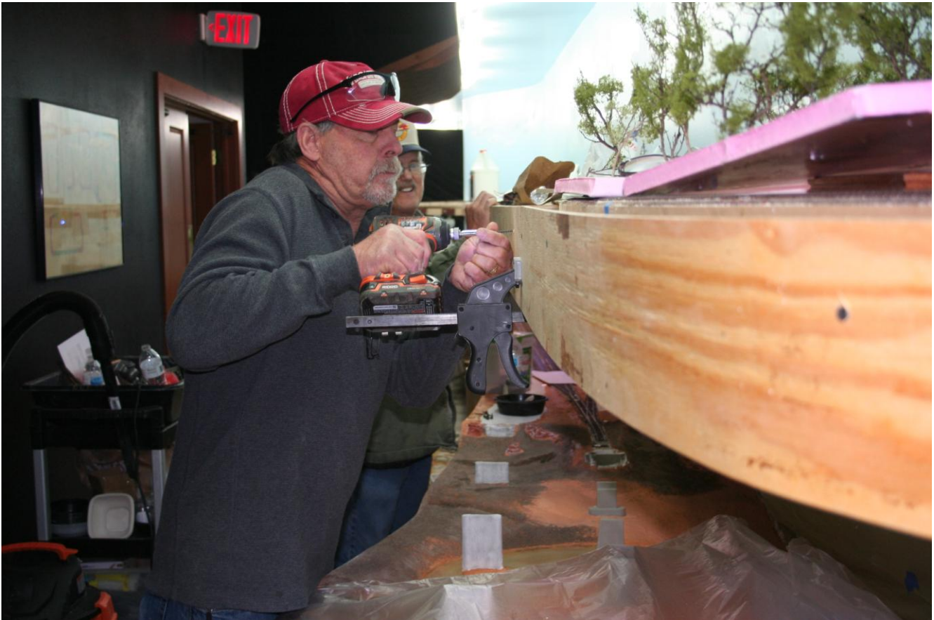
April 13,2019: New member Chris Mitchell assisting Tracy in installation of new fascia around the upper level above the Canadian River scene..
